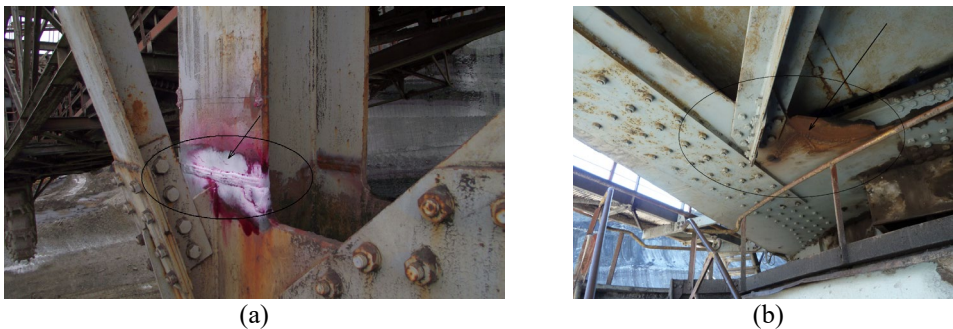
Fig.1 Cracks produced at (a) pillar base, (b) turntable
