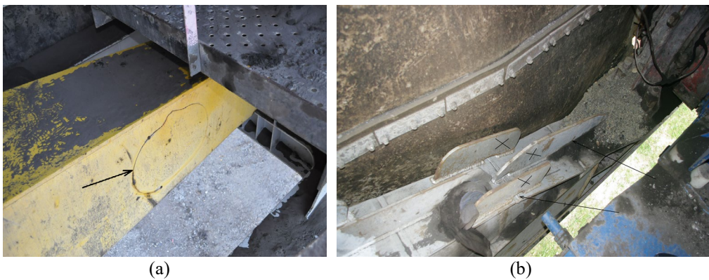
Fig. 5 Cracks at cup wheel reducer torque arm
